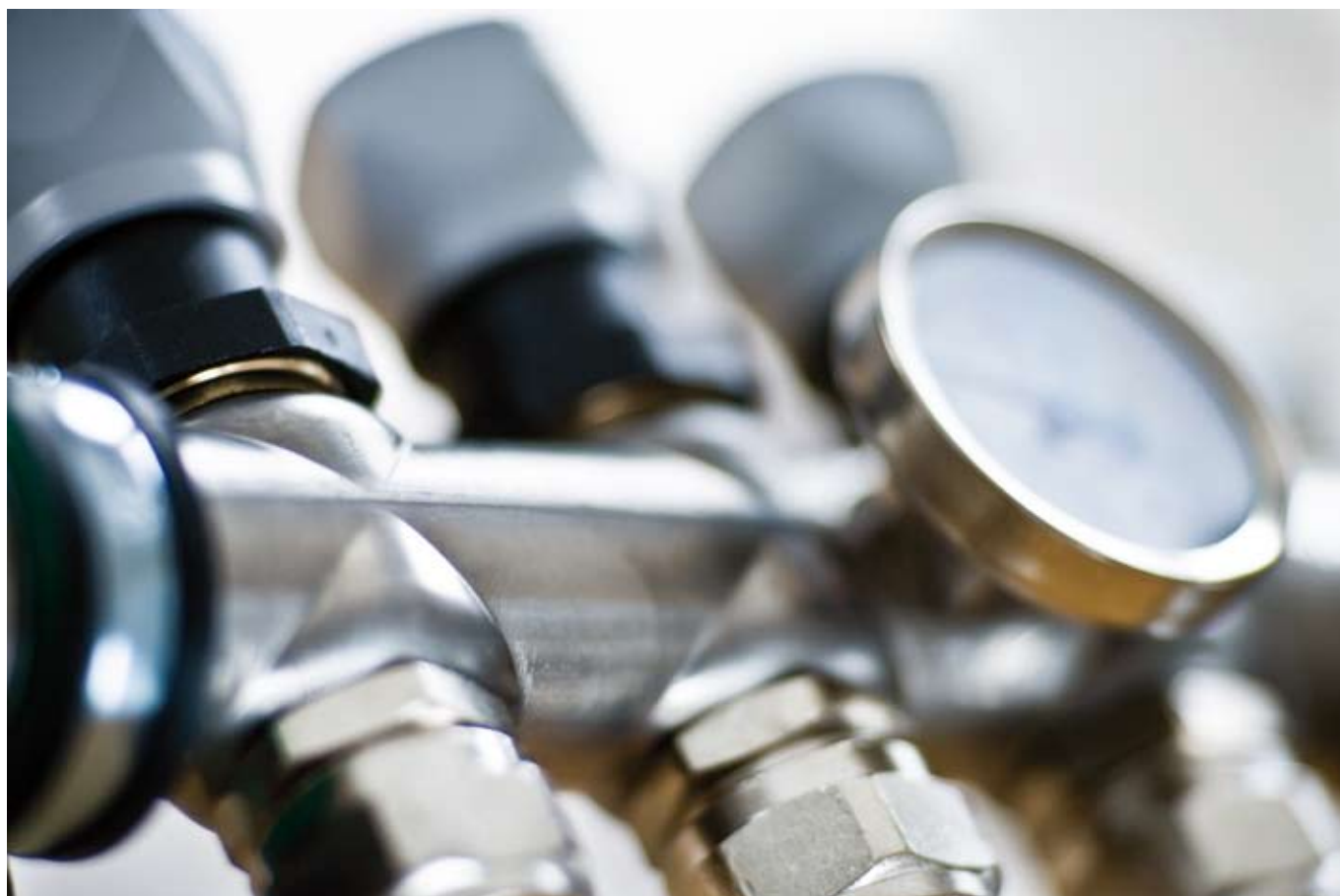
Thermotech Underfloor heating manifold
