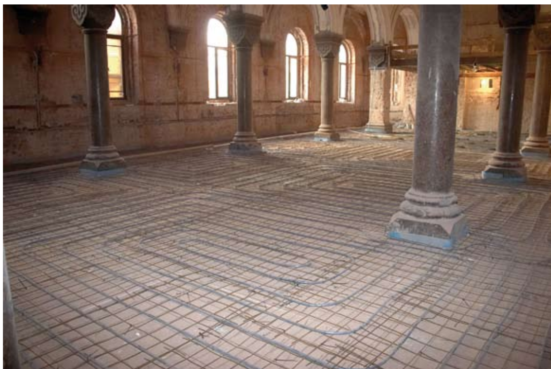
Installation of slab-on-grade concrete system, The Saint Andrey's Kritsky temple in St. Petersburg
